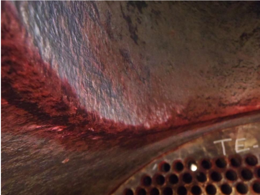
Inlet shell found heavily corroded
