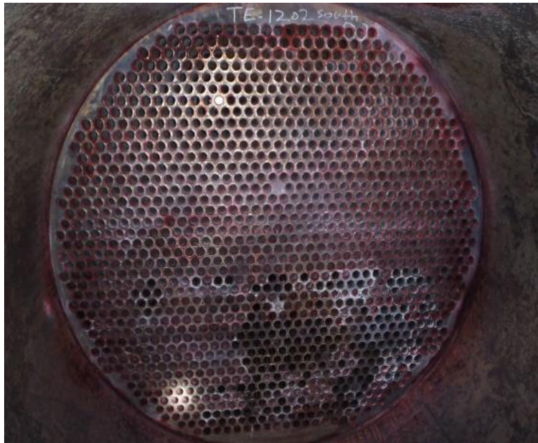
Severe Corrosion at tube Inlet side tube sheet
