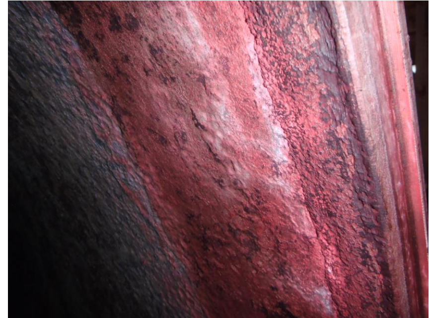
Inlet shell found heavily corroded
