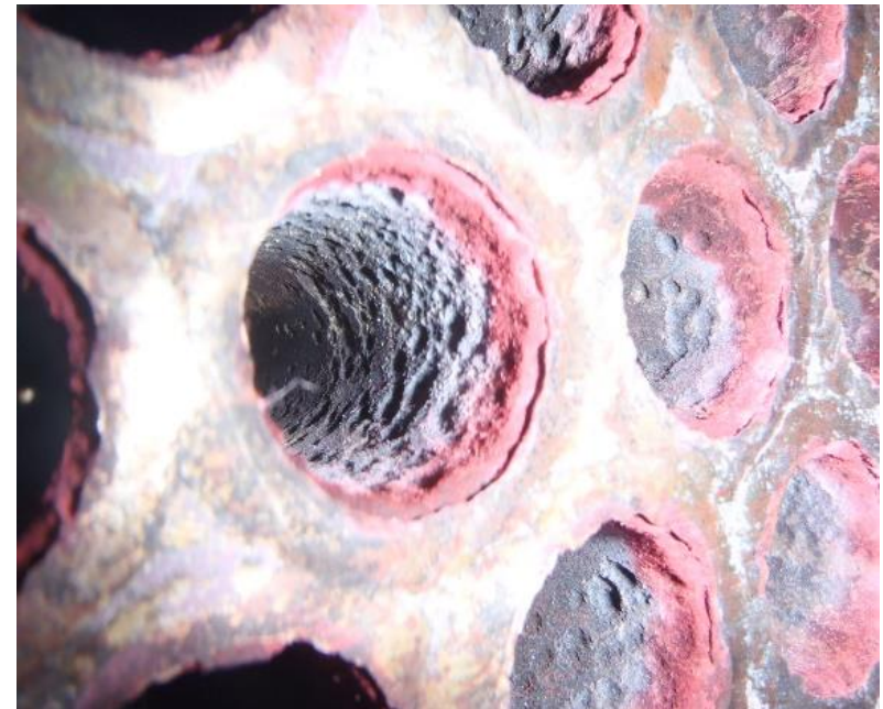
Deep pitting at tube inlet
