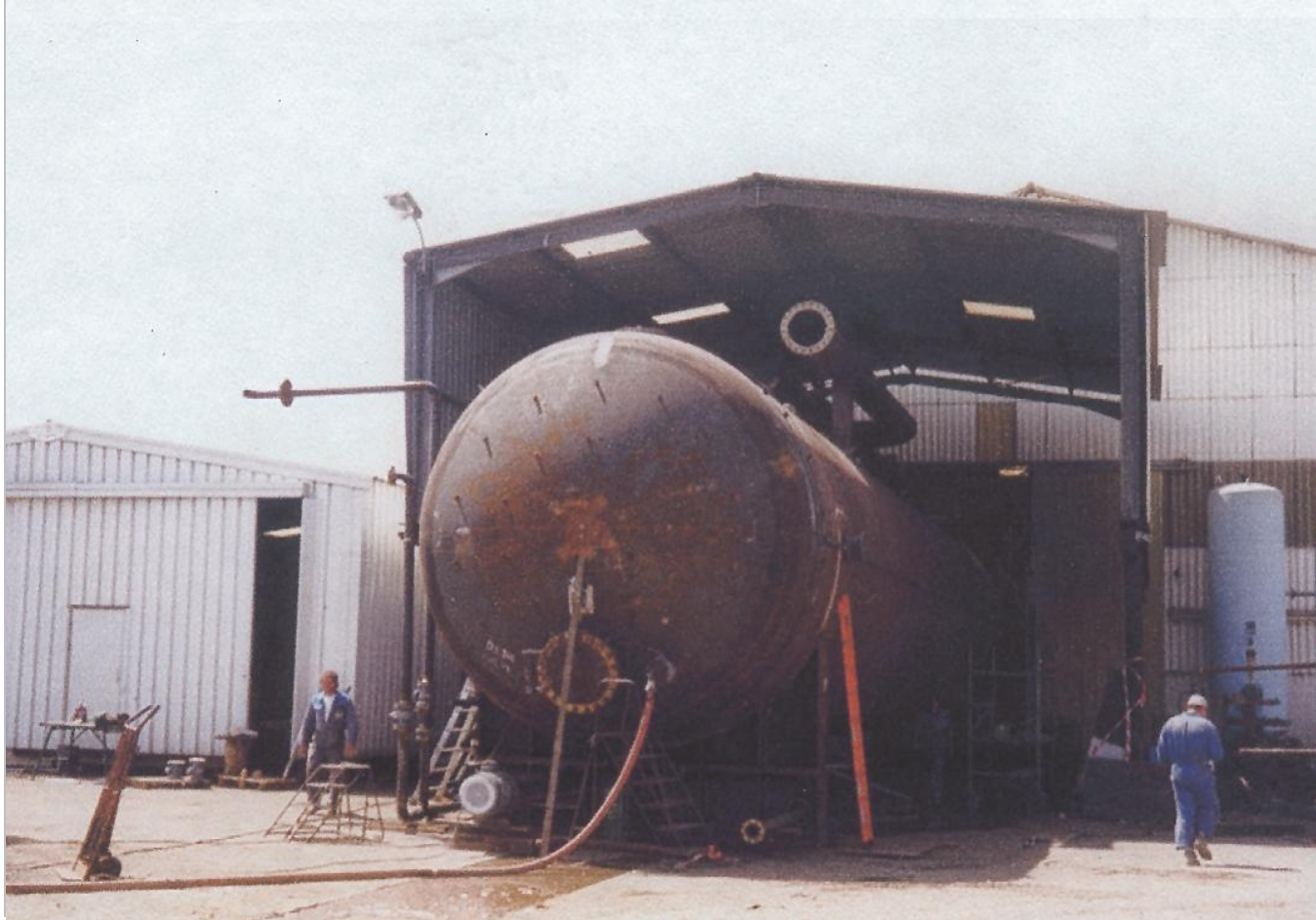
storage tank internal coated with SI14E
