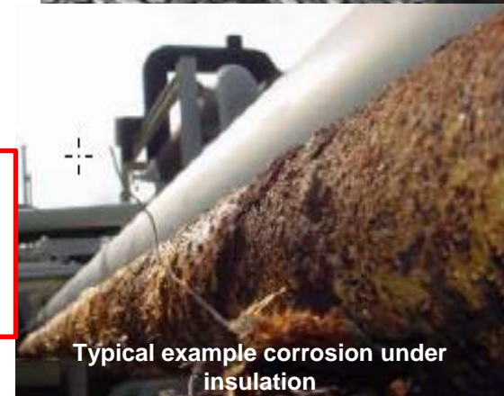
External stress corrosion cracking
