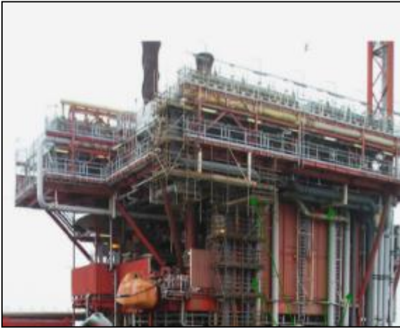
Gas - Condensate Pipework operating at temperatures up to 115C
