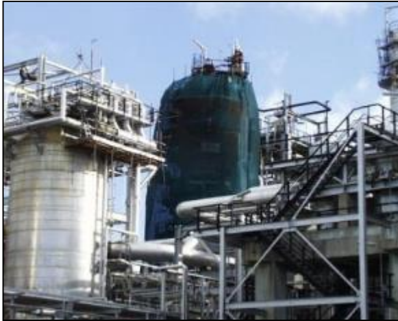
De-Asphalting Column in service with operating of 120 C
