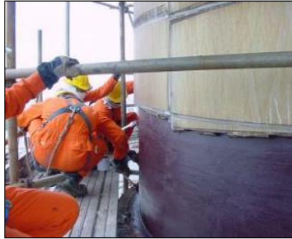
Surface preparation carried out using scrapers to remove loose rust to ST2 finish
