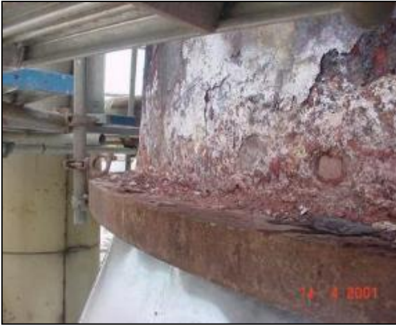
Fractionator Tower T102 in service operating at 120C
