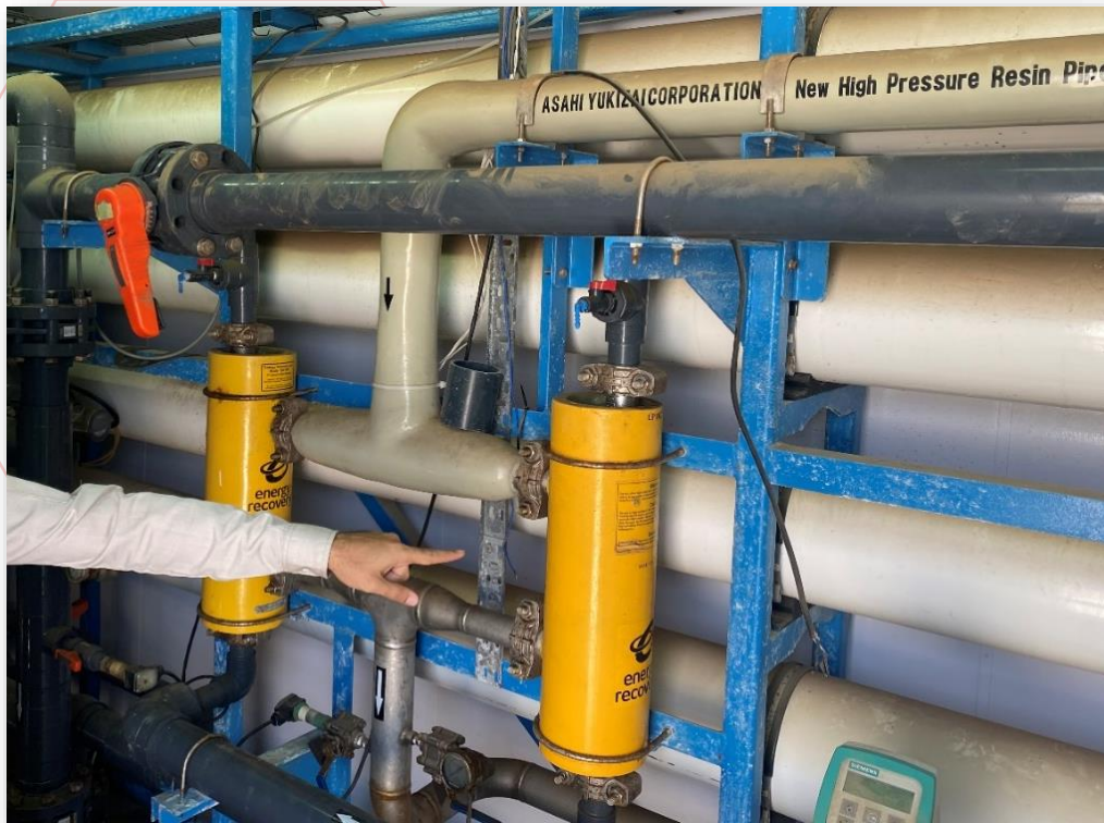
HPRP pipe installed in RO Plant for 80 bar pressure, 1 yr.
