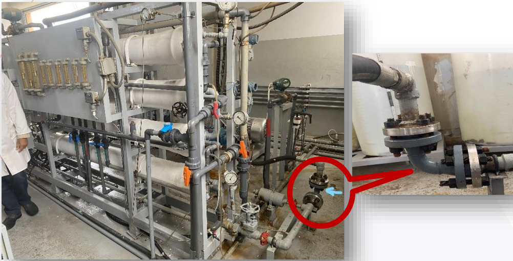
Hybrid spool under test in DTRI pilot plant at 70 Bar pressure
